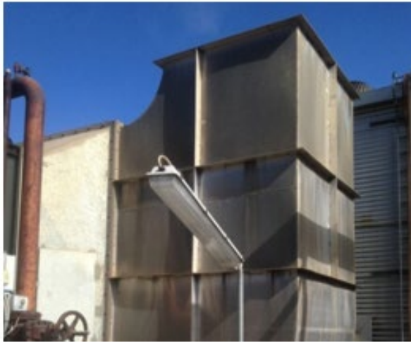
Vacuum Pump 9 (Paper Machine Hood Vent Exhaust)
