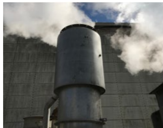
Vacuum Pump 7 – (794 First Bottom)
