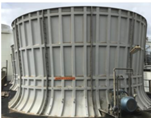
Cooling Tower (#1 Paper Machine Side)
