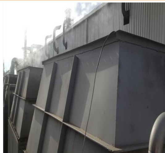
Vacuum Pump 10 (Paper Machine Hood Vent Exhaust)
