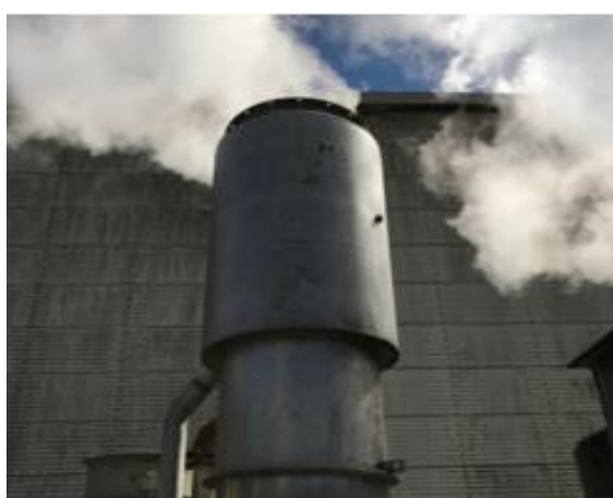
Vacuum Pump 7 - (794 First Bottom)
