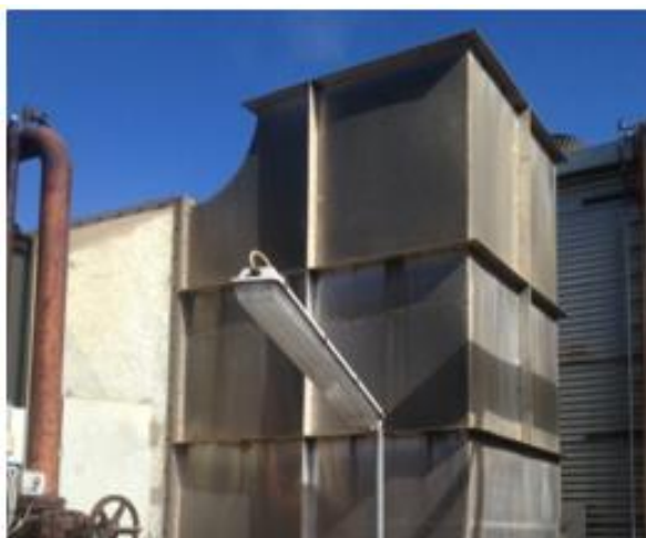
Vacuum Pump 9 (Paper Machine Hood Vent Exhaust)
