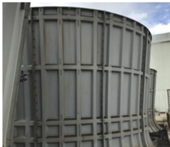
Cooling Tower (#2 Paper Machine Side)
