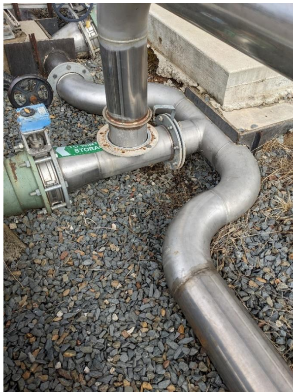
The modified valve system that prevents discharge of untreated wastewater from site following the Sandy Creek incident in October 2022
