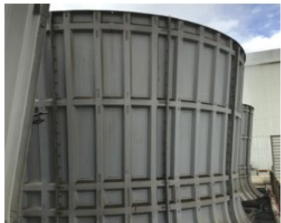
Cooling Tower (#2 Paper Machine Side)
