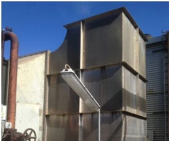
Vacuum Pump 9 (Paper Machine Hood Vent Exhaust)
