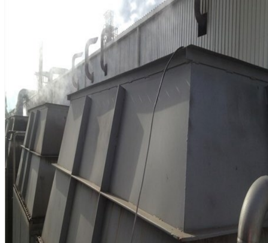
Vacuum Pump 10 (Paper Machine Hood Vent Exhaust)
