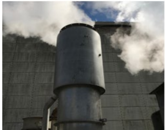
Vacuum Pump 7 – (794 First Bottom)
