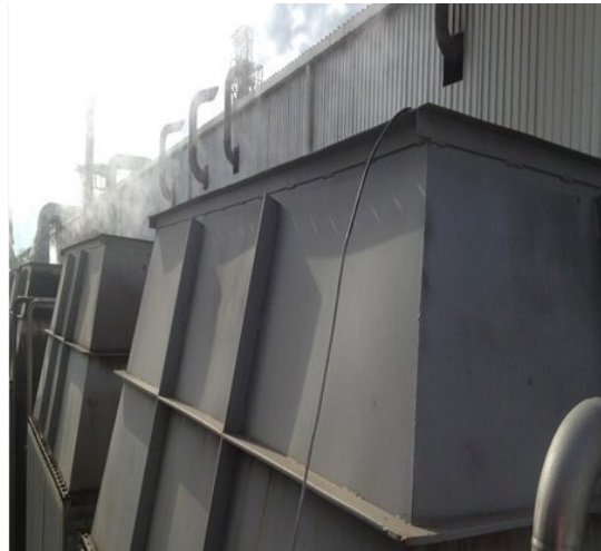
Vacuum Pump 10 (Paper Machine Hood Vent Exhaust)
