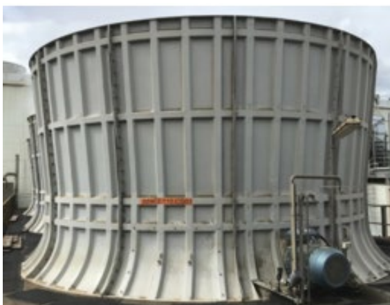
Cooling Tower (#1 Paper Machine Side)
