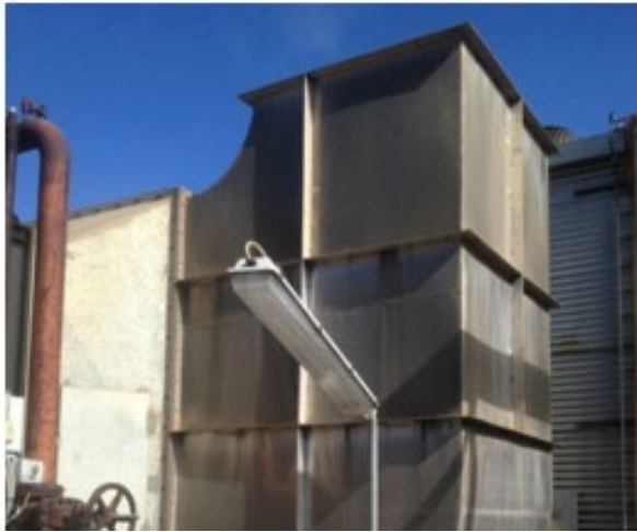
Vacuum Pump 9 (Paper Machine Hood Vent Exhaust)
