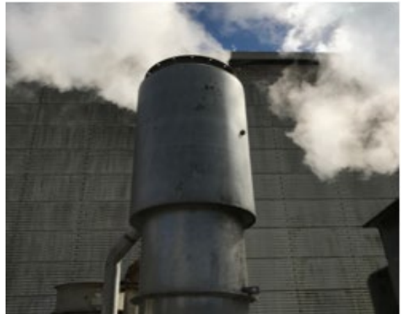
Vacuum Pump 7 – (794 First Bottom)
