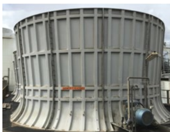
Cooling Tower (#1 Paper Machine Side)
