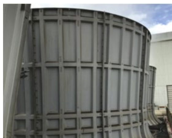
Cooling Tower (#2 Paper Machine Side)
