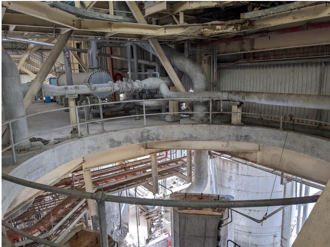
Parts of the paper production line have been removed for use on Visy premises elsewhere during the site's extended shutdown
