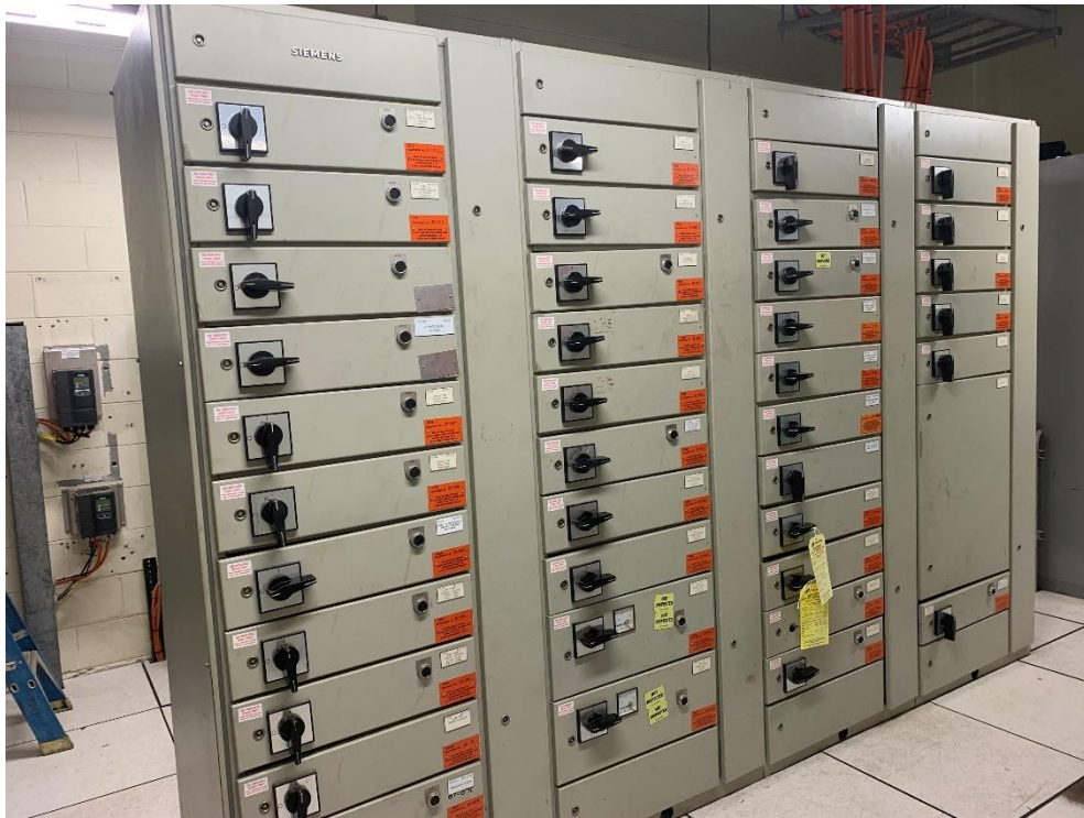
Switchboard indicating most processes in 'off' position
