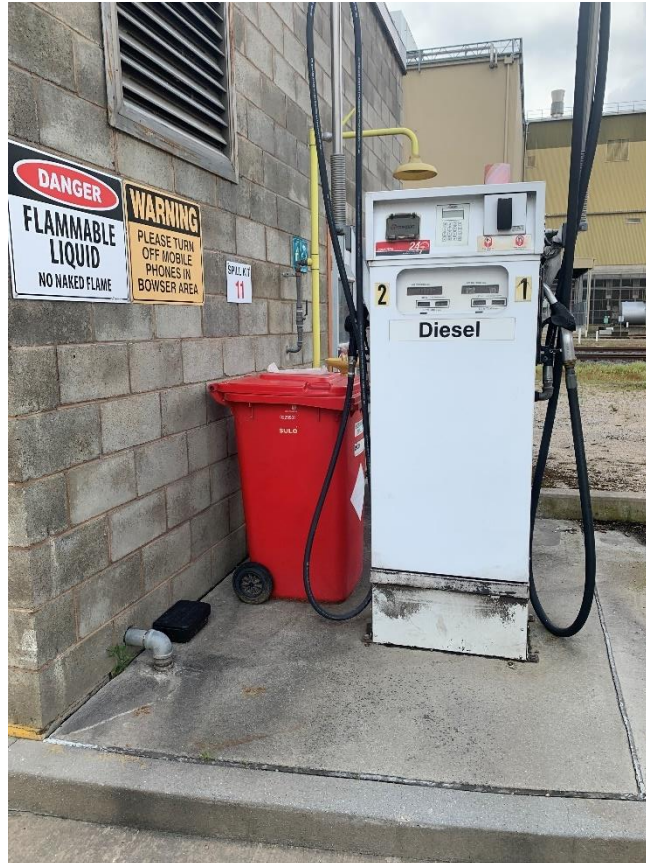
Dangerous goods and safety signage at diesel bowser, fully stocked spill kit adjacent
